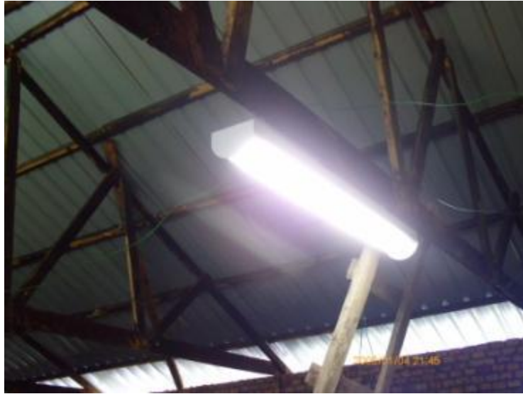
One of the light bulbs turned on
